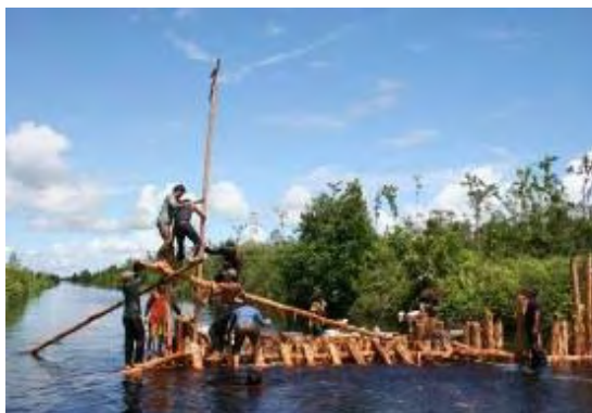
Figure 9.4: Peatland restoration Blocking of a canal in degraded peat swamp forests in Central Kalimantan, by local communities using manual traditional techniques. (Photo: Marcel Silvius, Wetlands International).
