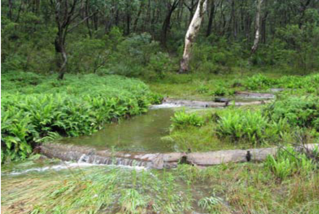
Figure 10.1 – Coir logs used to decrease water velocity and repair an eroded section of swamp
